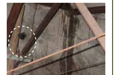
What is left of the electric light inside
